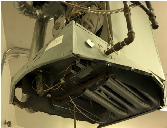
Figure 1: Damaged unit heater Potentially caused by failed Vent System
