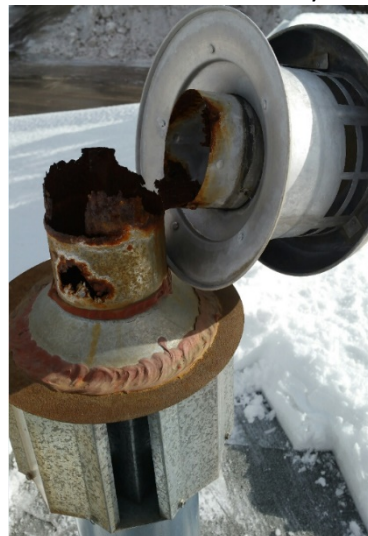
Figure 2: Failed Concentric Vent System
